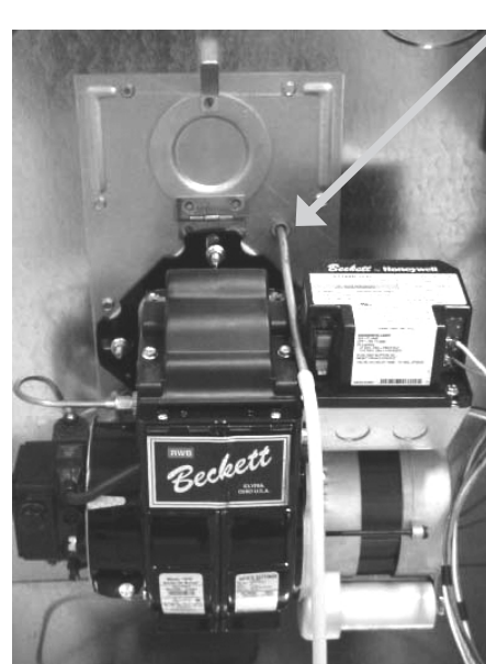
Over-fire draft access port.
